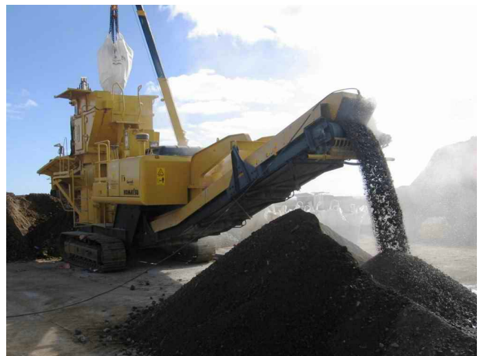
Purpose built soil blender mixes up to 500 MT per day
